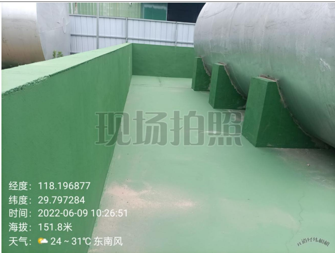
罐区废气收集、围堰及防渗
