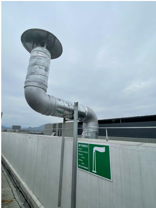
DA003 焊接烟尘排气筒
